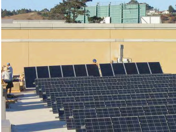
UNI-SOLAR framed modules and poly-Si modules at 30° tilt, on flat roof (SPF)
