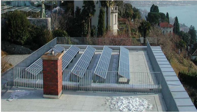
One of many 20-30° tilted poly and mono-Si roof systems monitored by ISAAC in same region
