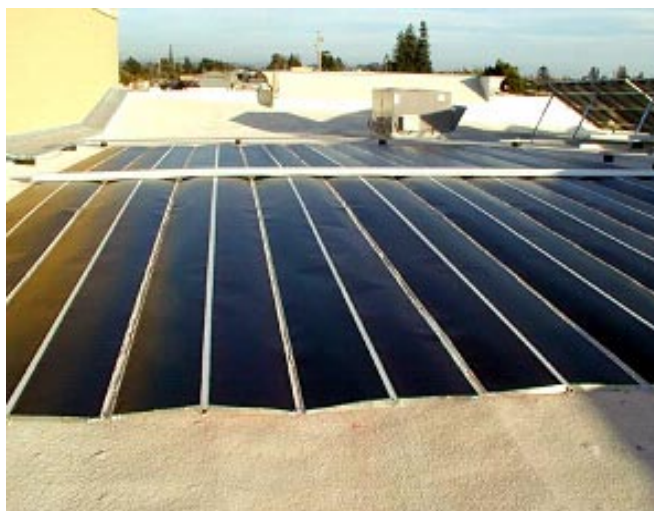
UNI-SOLAR laminates at < 3° tilt, on membrane roof (SPF)
